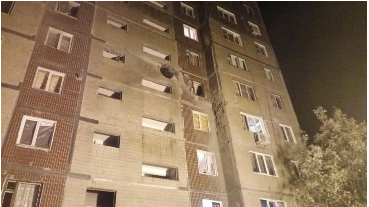
Fig. 7 – Traces from the shell hit in the residential building at 10, Stroitel residential quarter.
