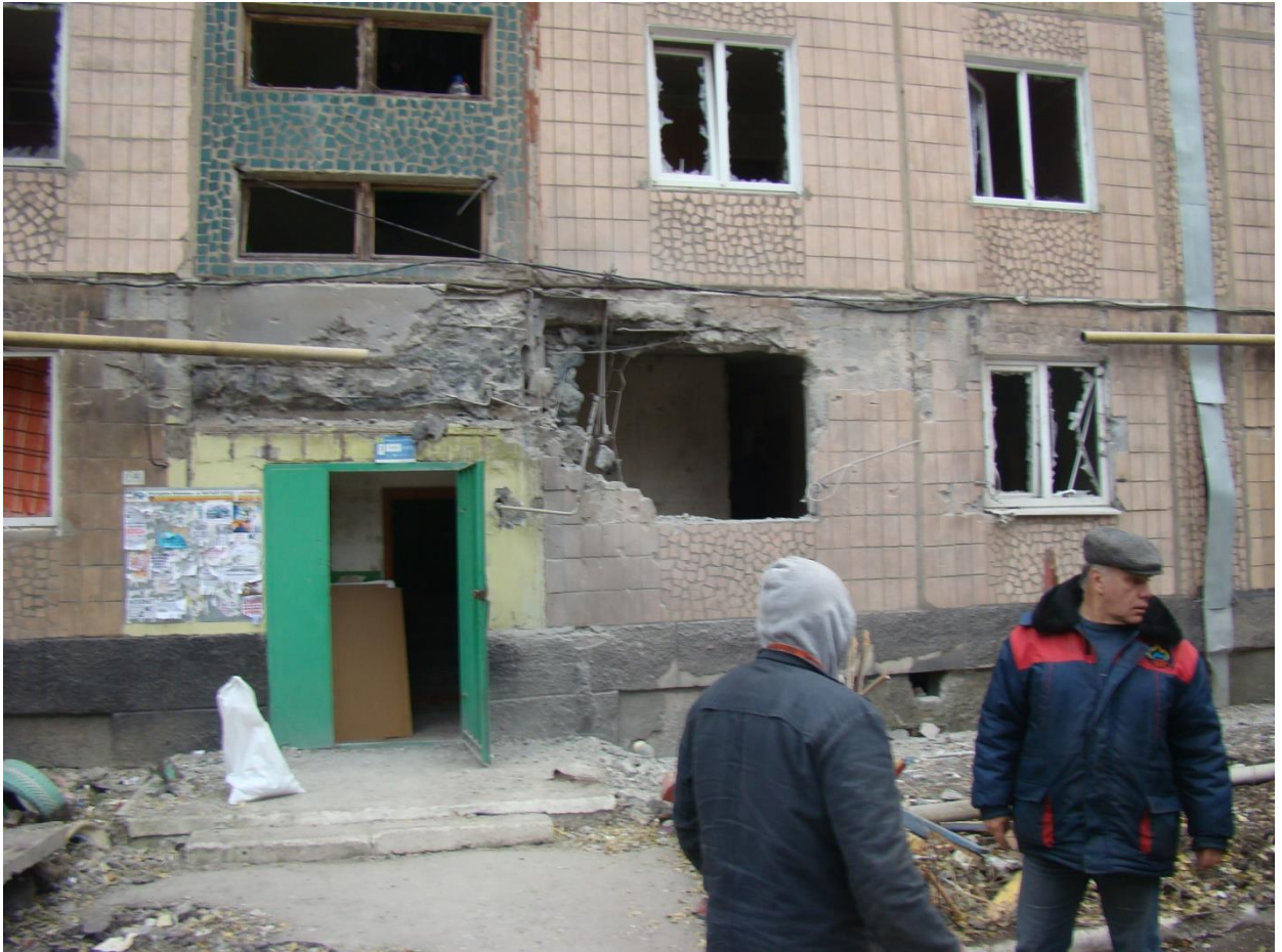
Fig. 8 – Traces from the shell hit in the residential building at 7, 50th anniversary of the USSR formation Str.
