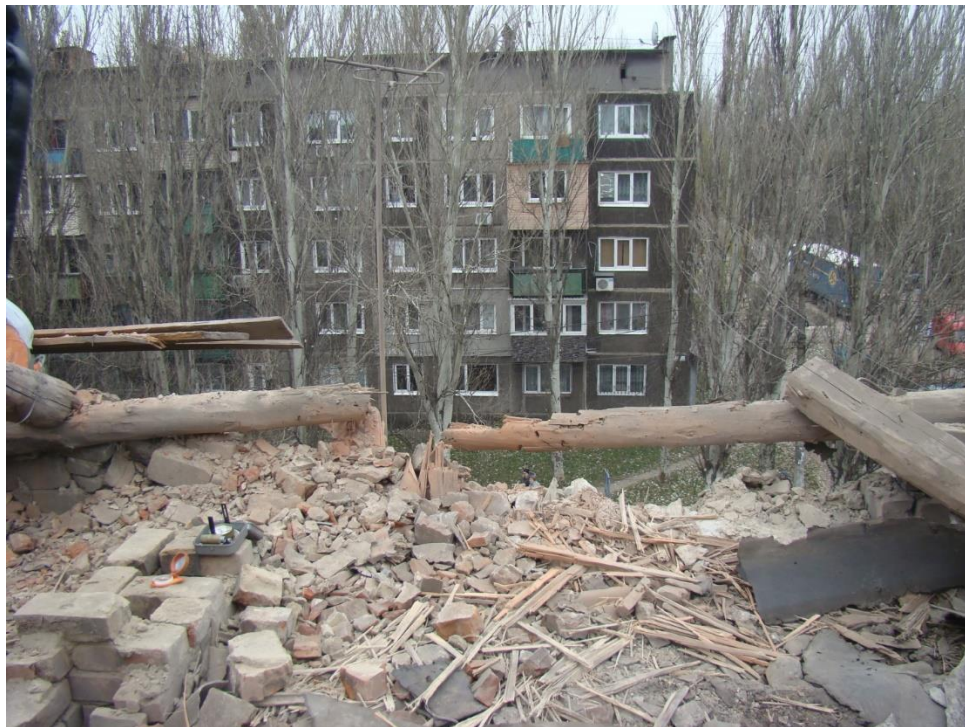
Fig. 9 – Damaged roof of the residential building in 40/73, Heroes of Stalingrad St., Makeyevka.
