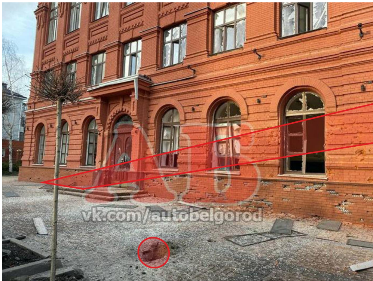
Fig. 28 - The crater and the trace from the main flow of fragmentation scatter in the case of shell hit 5.
