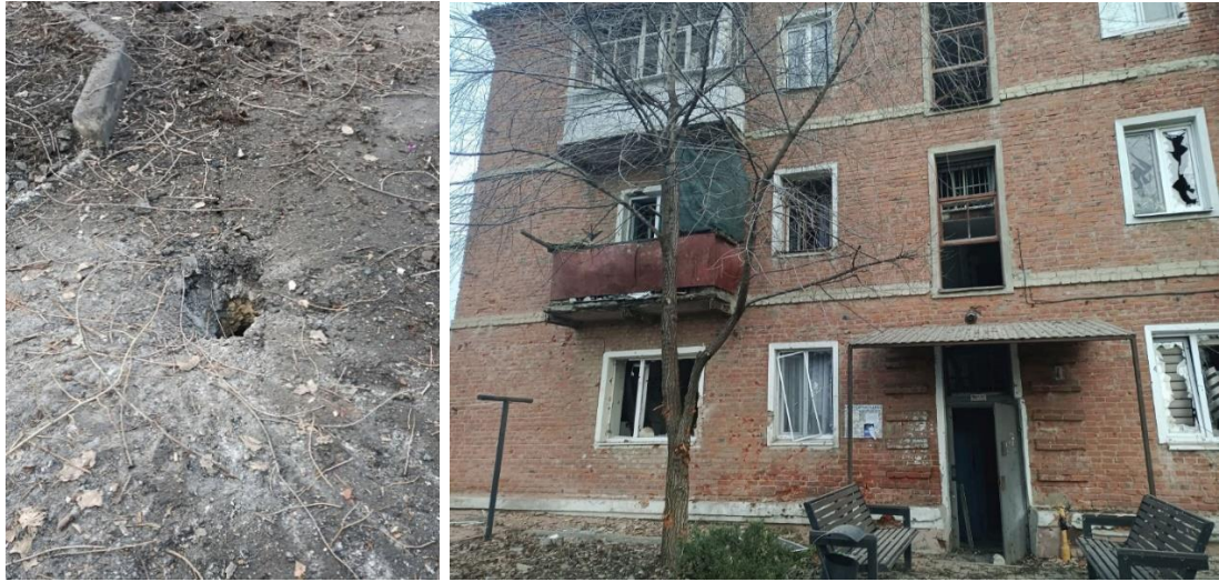
Fig. 4 - Shell hit at 2 Second Kotlozavodskiy Lane. 18
