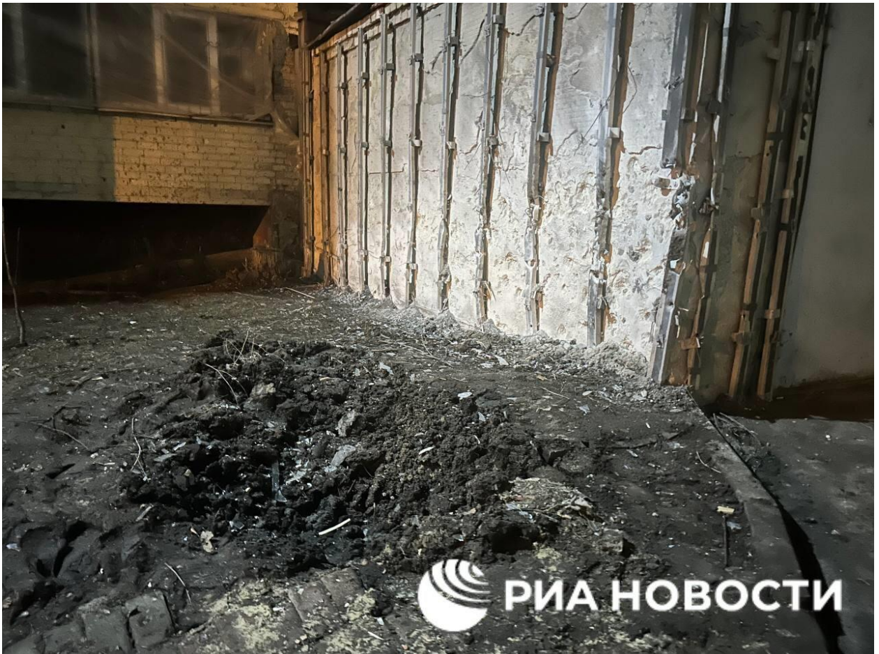
Fig. 18 – A crater near residential building at 39, Slavy Avenue. 35
