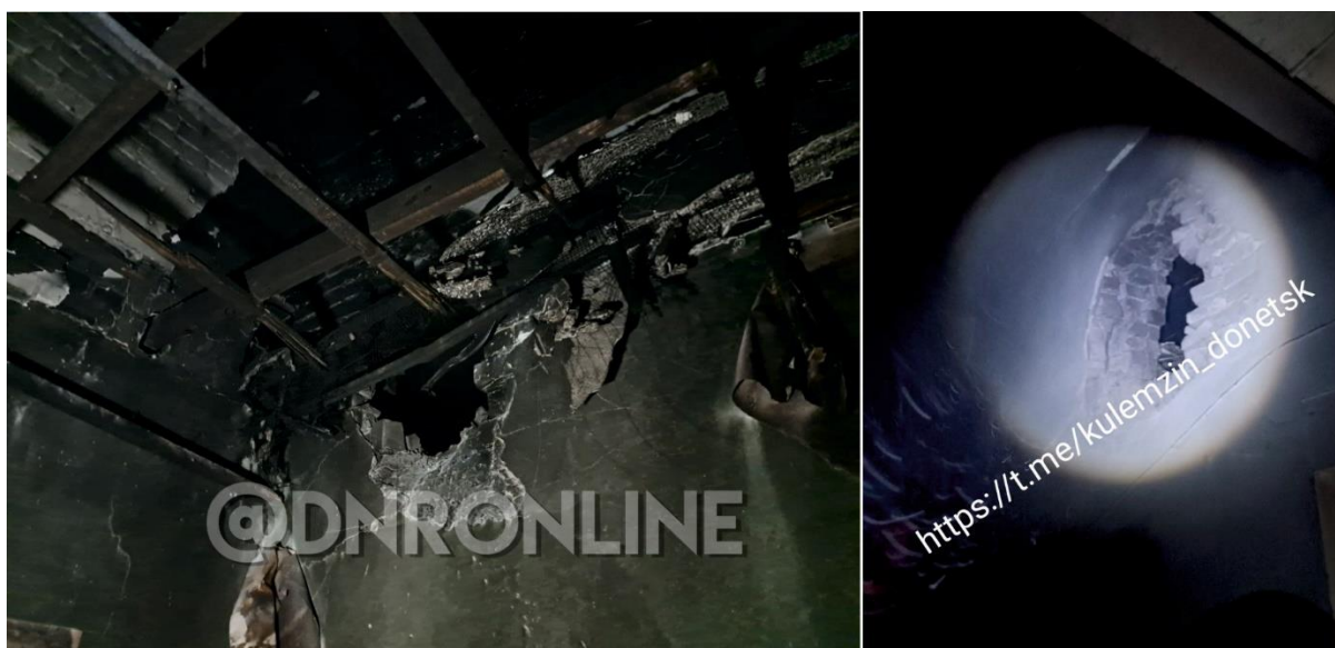
Fig. 19 – Walls damaged in the sports and recreation complex the M. Gorky DoNMU due to the shell hit on December 19, 2022. 48 49
