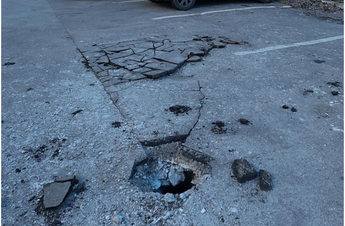
Fig. 10 – A camouflet near the DoCTMA building No. 12 after the shelling on December 18, 2022
