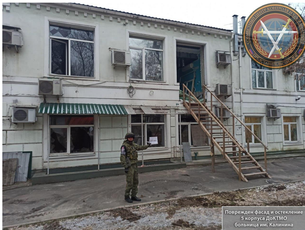
Fig. 12 – Damaged façade and glazing on the eastern side of the DoCTMA building No. 5 after the shelling on December 18, 2022 45
