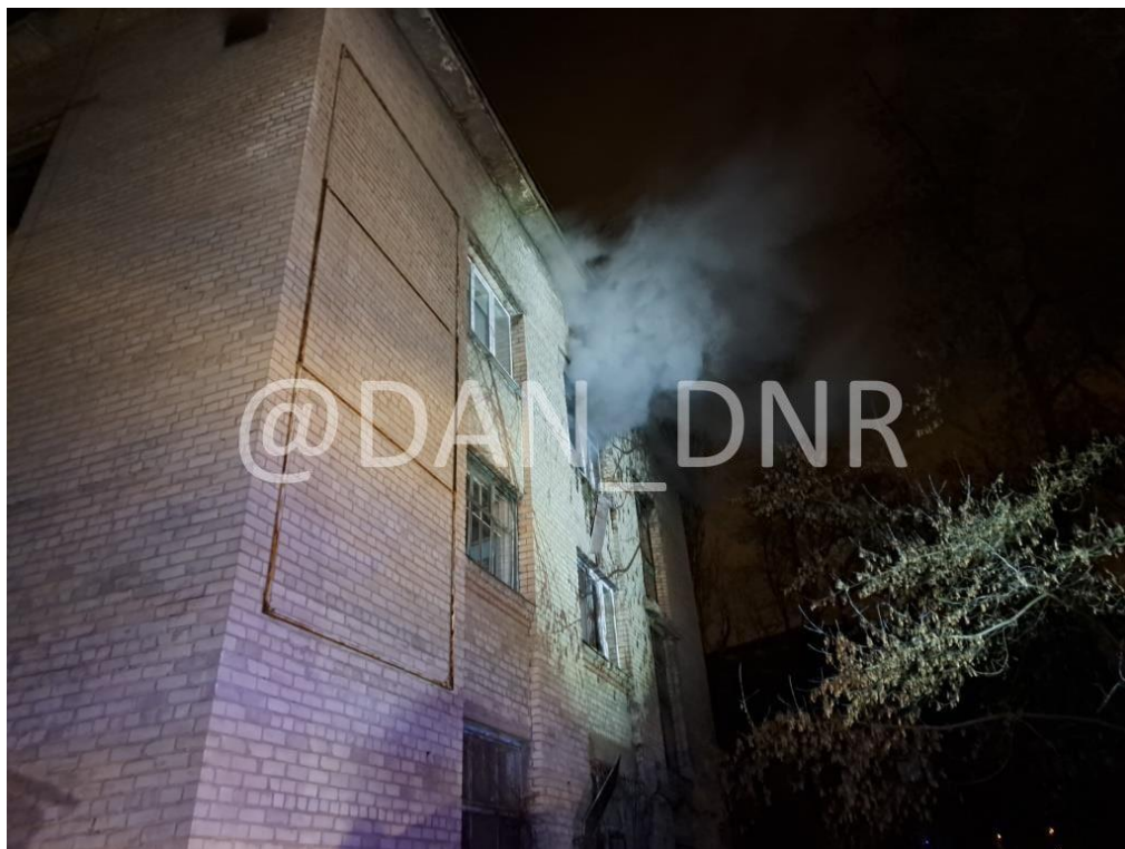
Fig. 18 – Fire outbreak in the sports and recreation complex of the M. Gorky DoNMU M. due to the shell hit on December 19, 2022. 47
