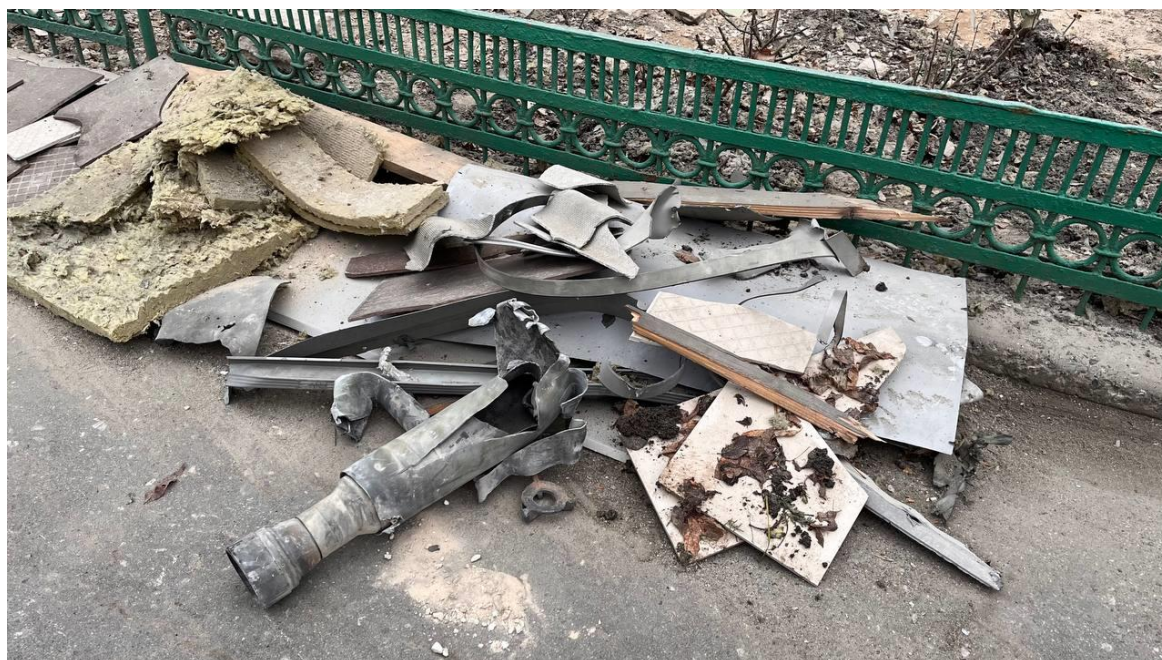
Fig. 13 – A fragment of the propulsion unit salvaged after the shelling from under the rubble of the DoCTMA building No. 6 on December 18, 2022 46
