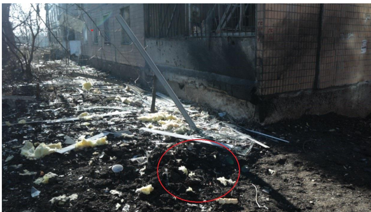
Fig. 32 – A shell crater next to the residential building at 6, Kapitana Ratnikova St., after the shelling on December 19, 2022
