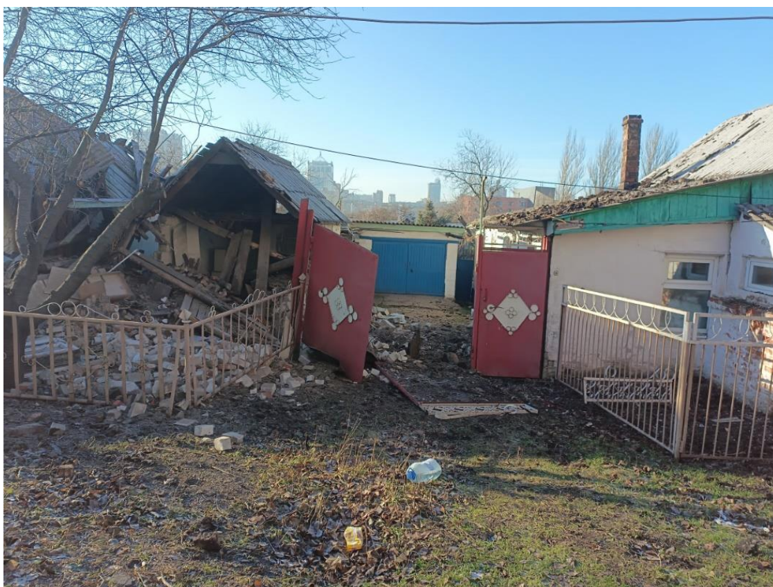
Fig. 29 – Direct shell hit in the residential building at 5, Barvenkovskaya St., due to the shelling on December 19, 2022
