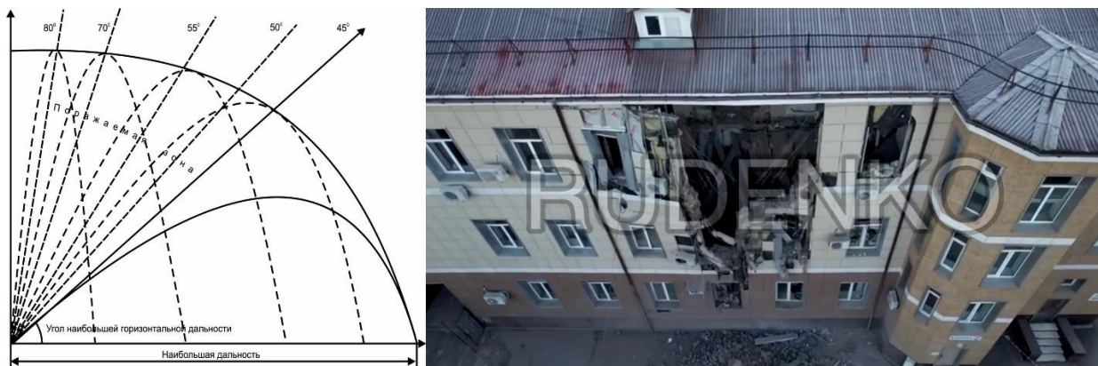
Fig. 53 – Left: flight path-angle of departure dependence 64 ; right: the consequences of hitting the Grad MLRS projectile in DoCTMA building No.10 65 .
