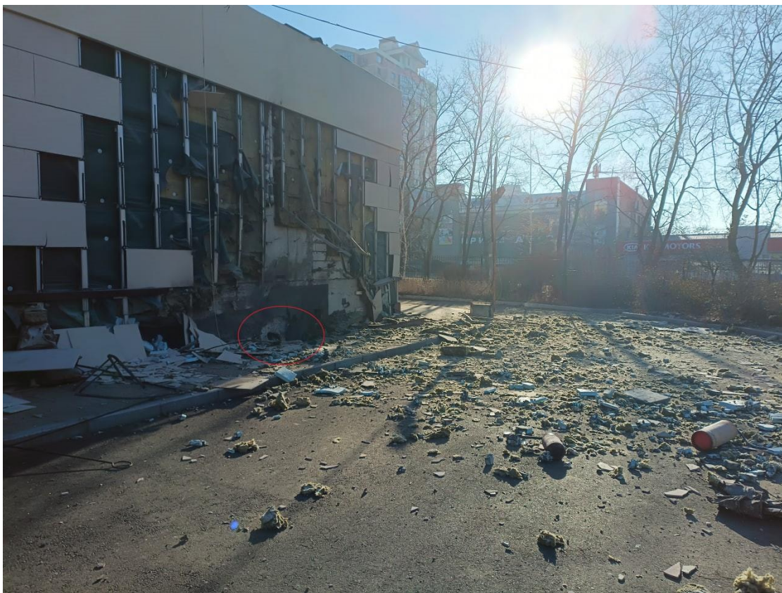
Fig. 28 – Shell hit into the DoCTMA building No.15 on December 19, 2022
