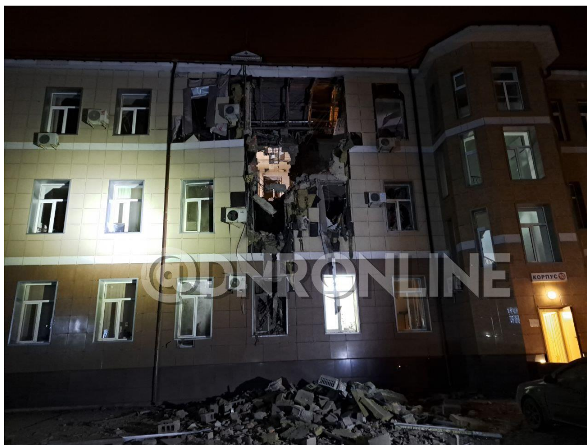
Fig. 25 – Direct shell hit in the DoCTMA building No.10 on December 19, 2022. 53
