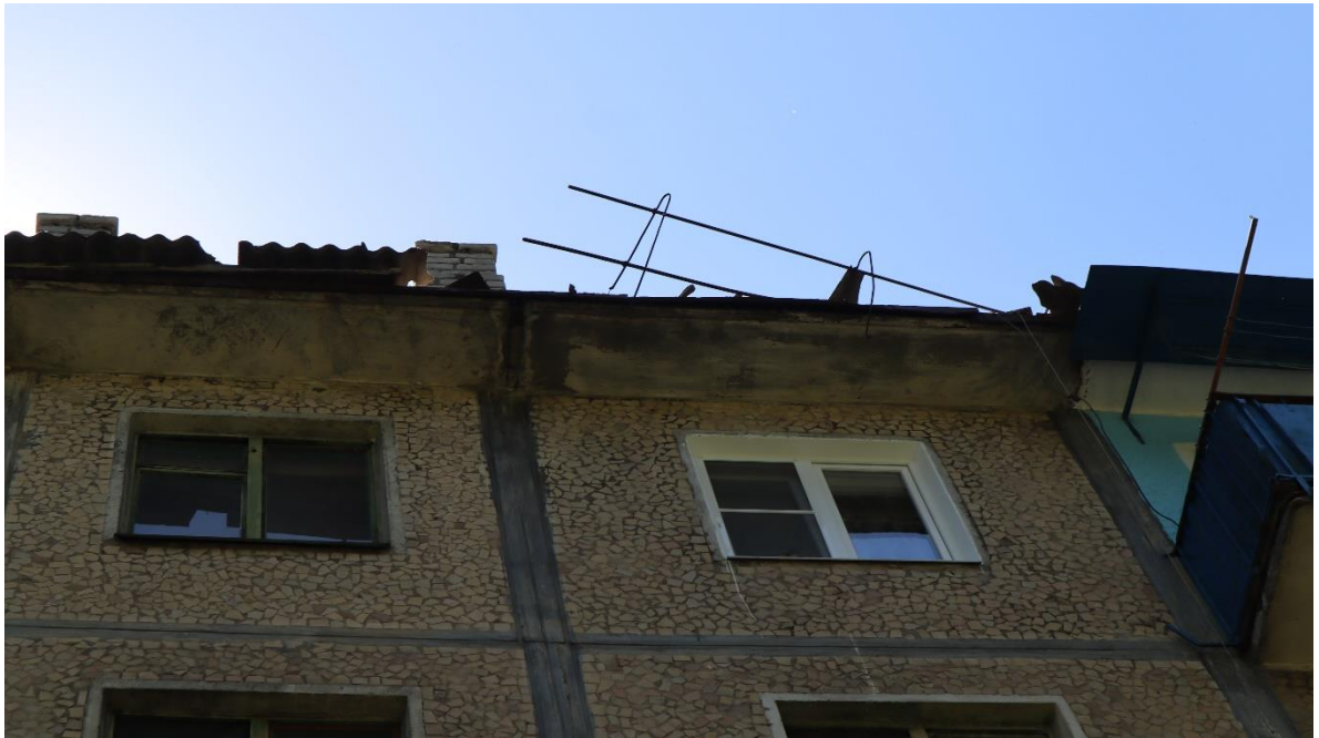
Fig. 9 - The second trace of the FSM detonation on the roof of the residential building No.13.
