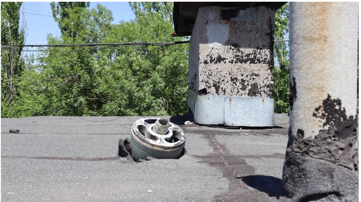
Fig. 12 - Debris of the cluster warhead frame on the roof of the residential building No. 18 in Shakhtyorskiy Quarter.
