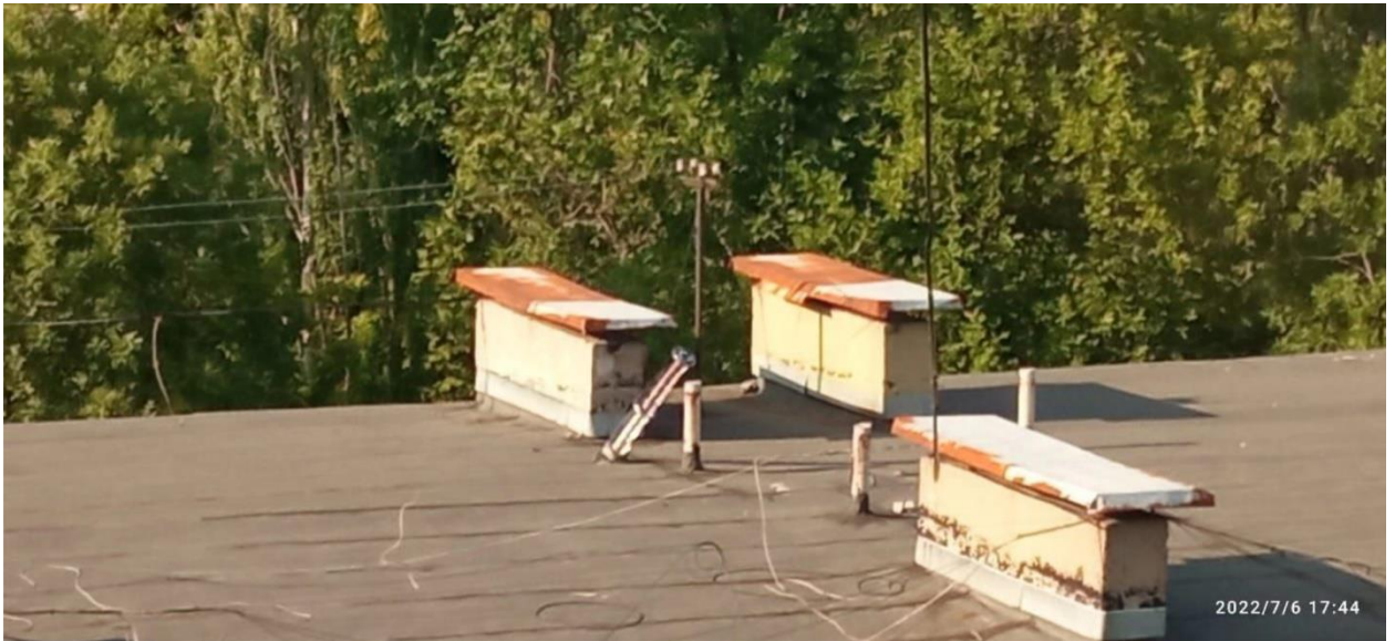
Fig. 11 – The cluster warhead frame protruding from the roof of the residential building No. 18.
