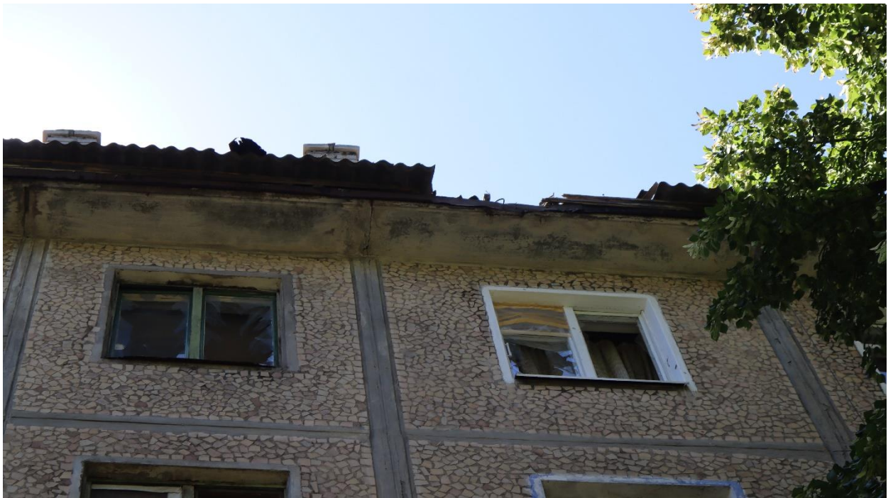
Fig. 8 – The first trace of the FSM detonation on the roof of the residential building No. 13
