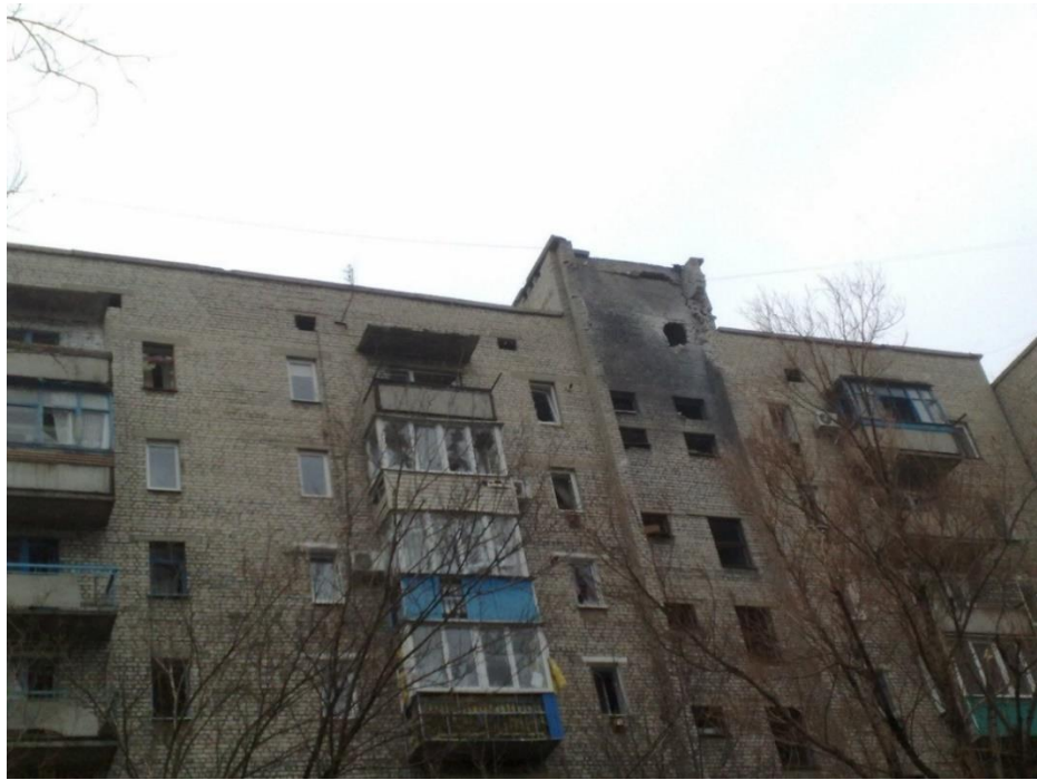
Fig. 21 – The through hole in the wall of the residential building as a result of shell hit 9 39 .
