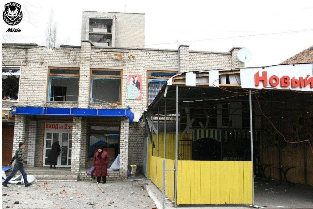
Fig. 7 – The roof of the Kirovchanka consumer services center damaged by shell hit 4 28 .
