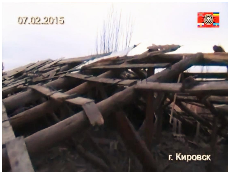
Fig. 12 – The roof damaged by shell hit 6 31 .
