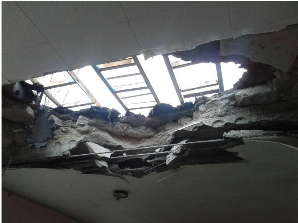
Fig. 3 – The through hole in the roof of the kindergarten as a result of shell hit 2 25 .
