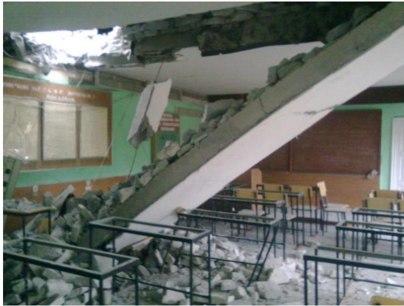
Fig. 17 – Ceiling of the training class in the technical college, which collapsed as a result of shell hit 7 36 .
