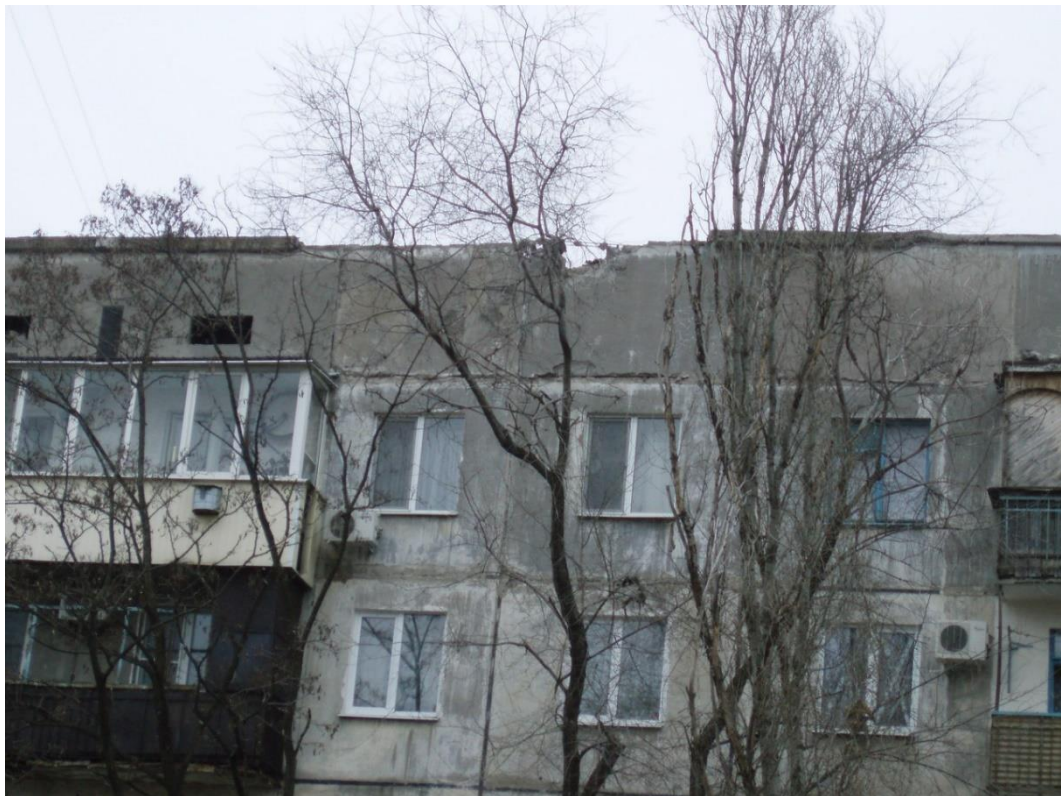
Fig. 6 – The roof damaged by shell hit 3 27 .
