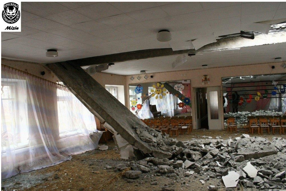
Fig. 4 -The ceiling of the music hall of the kindergarten collapsed as a result of shell hit 2 26 .
