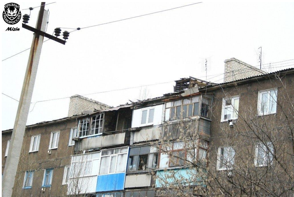
Fig. 11 – View of the roof destroyed as a result of shell hit 6 30 .
