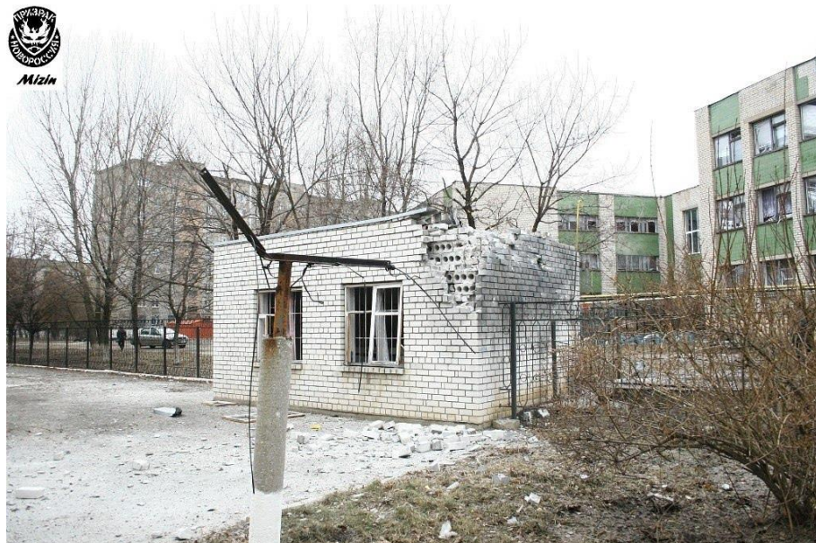
Fig. 2 – Destroyed eastern corner of the boiler station roof as a result of shell hit 1 24 .
