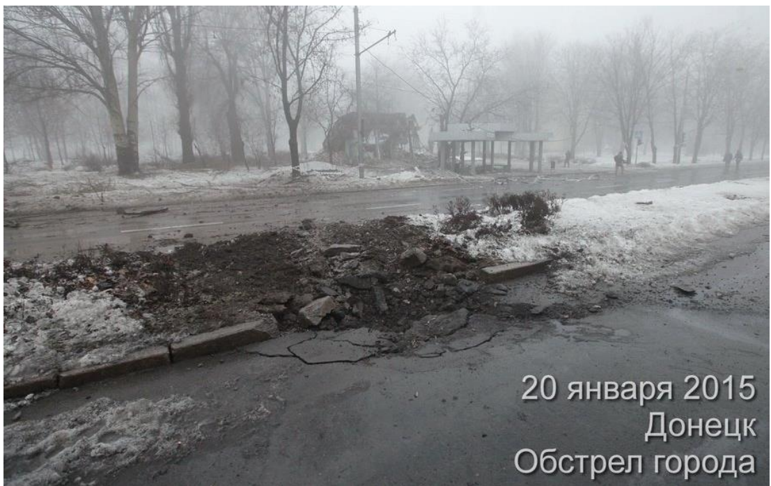
Fig. 13 - The shell hit into the median lane a bit south of Kievsky DEC public transport stop 49 .
