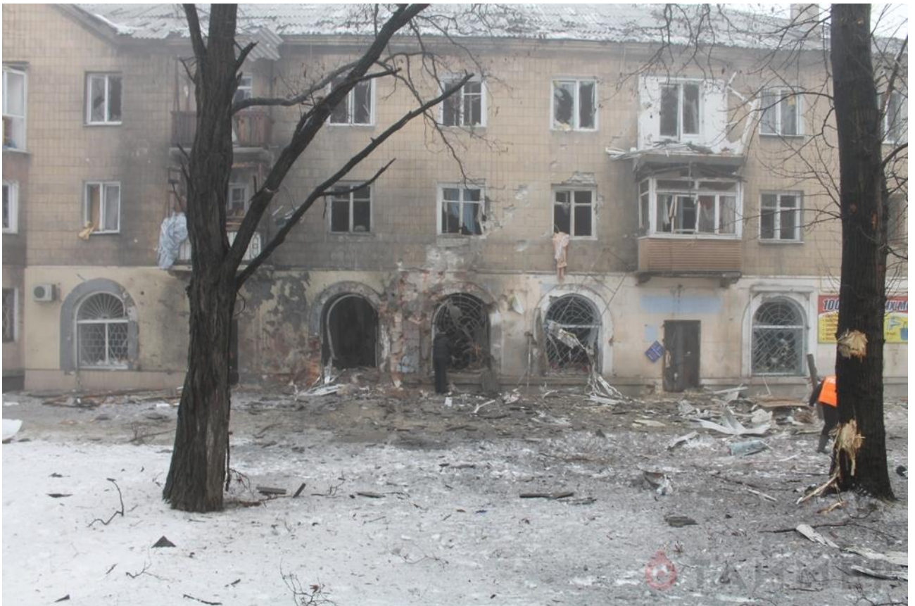
Fig. 15 – The shell hit into the base of the wall of the residential building in 21, Kievsky Ave 50 .
