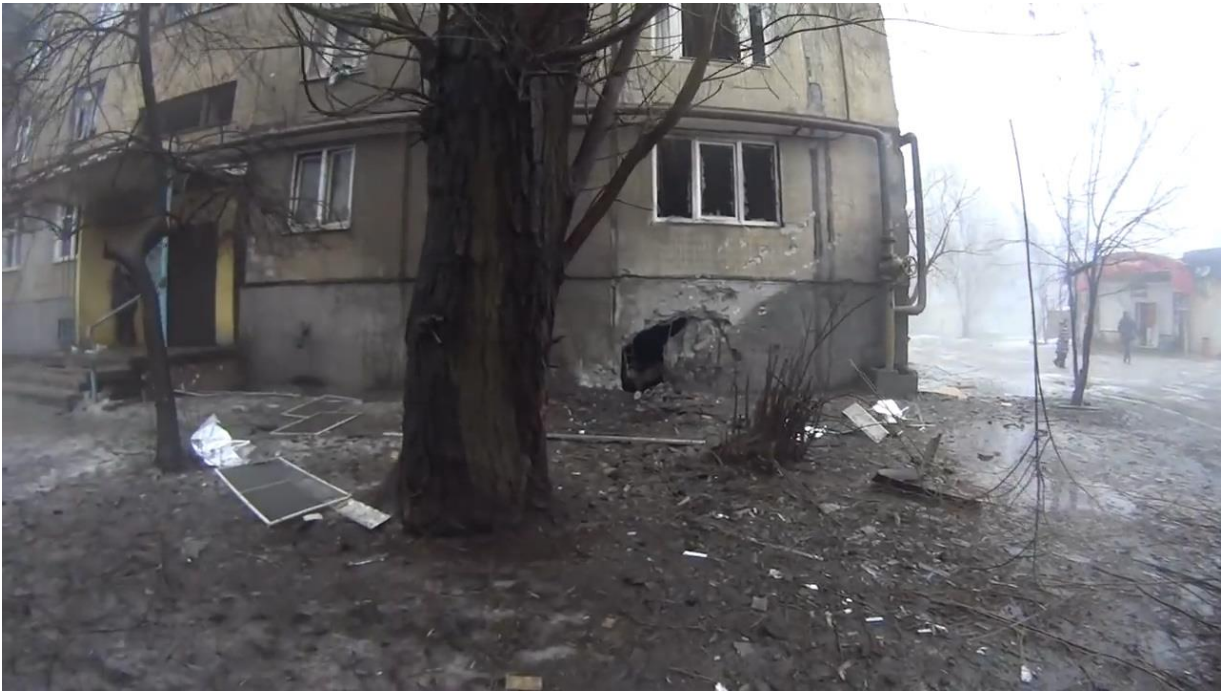
Fig. 8 – A trail from the detonation of a projectile at the wall base of the residential building in 3, Politboitsov St 44 .
