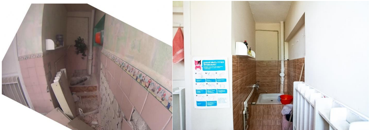
Fig. 16 – The technical niche in Nursery School No. 204: on the left - immediately after the shell hit (as of 20.01.2014) 51 ; on the right – after renovation (as of 20.08.2021).
