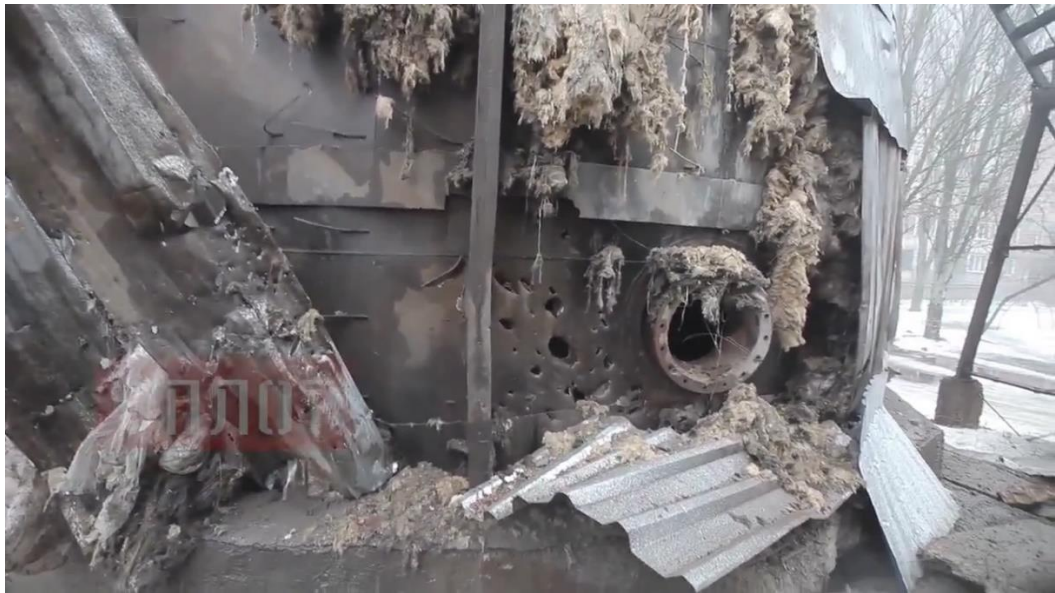
Fig. 5 – The technical tank of the boiler house damaged by explosion 41 .
