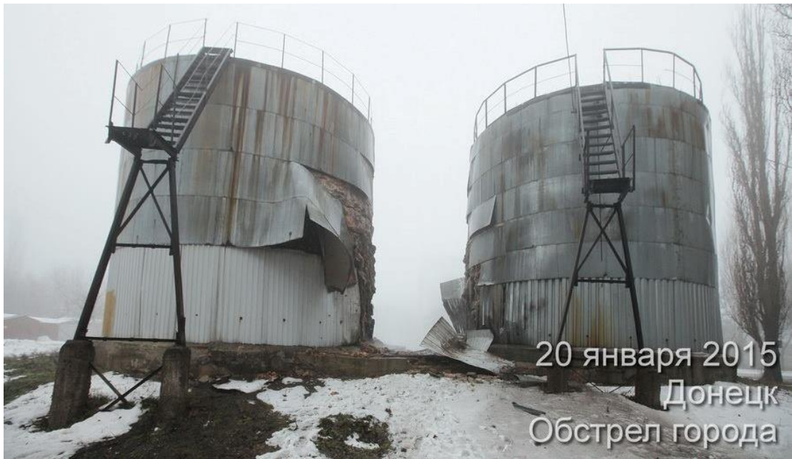
Fig. 6 – The technical tanks of the boiler house located nearby residential building in 10, Politboitsov St., Donetsk. The shell detonated between the tanks 42 .
