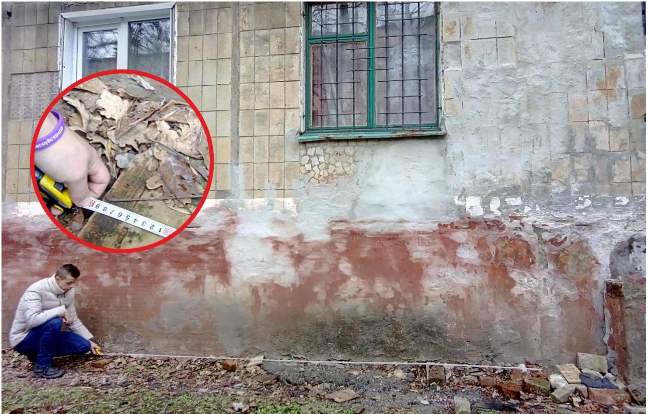
Fig. 21 - Measuring the width of traces of the main stream of fragments on the wall of the building, shell hit 5 (14.12.2021).
