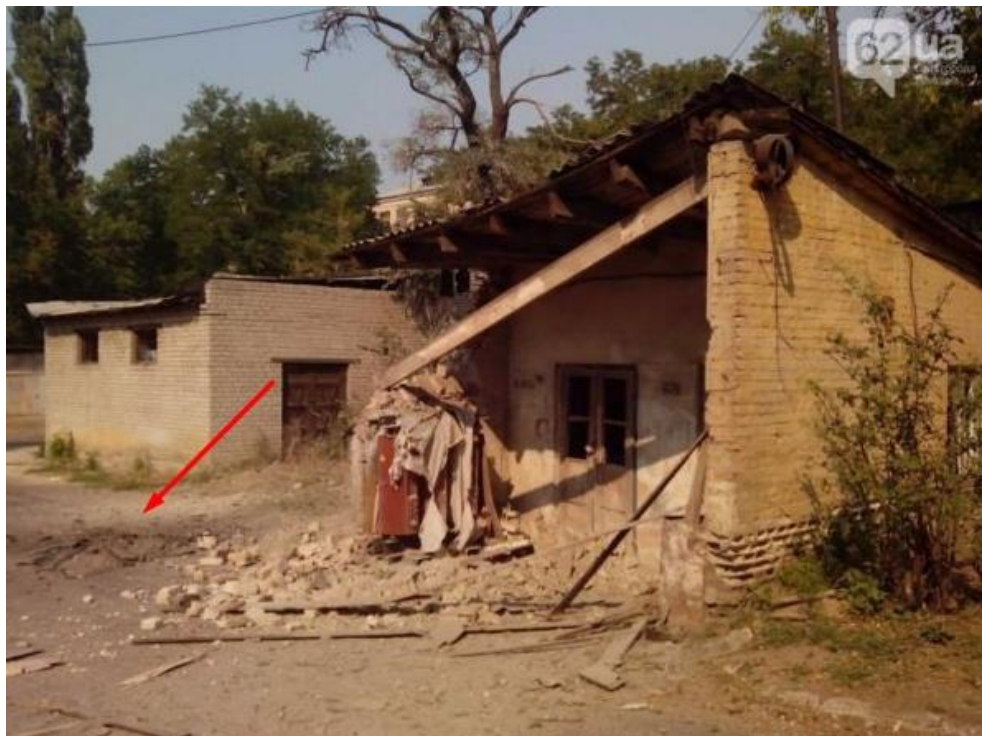
Fig. 9 – Shell hit (4) about 60 meters west of the south-east corner of the DonNTU educational building No. 2 38 .
