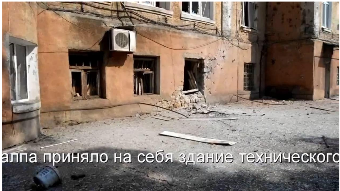
Fig. 8 – Shell hit (3) in the base of the western wall of the DonNTU educational building No. 2 37 .
