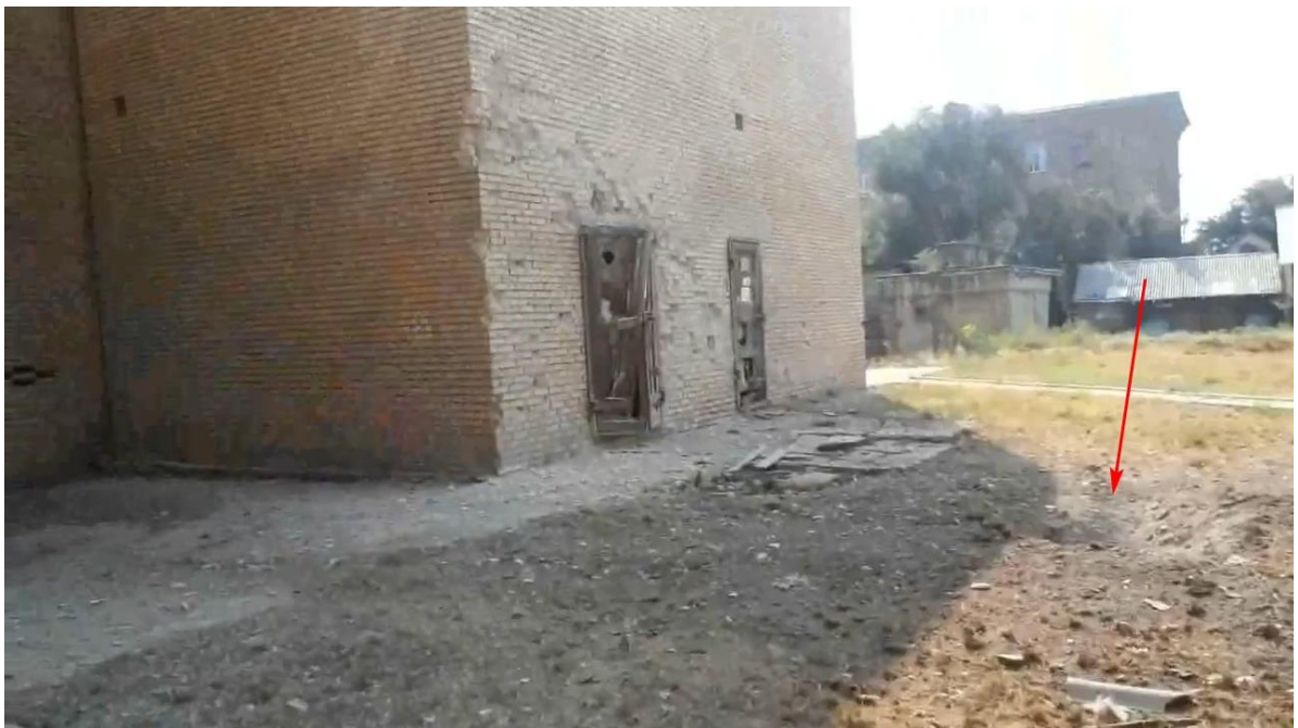
Fig. 17 – The trail of a shell hit (8) nearby the power substation of the DonNTU educational building No. 9 45 .
