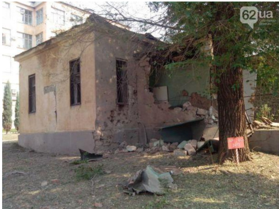
Fig. 14 – Shell hit 6 that destroyed the north-west corner of a one-story building 43 .
