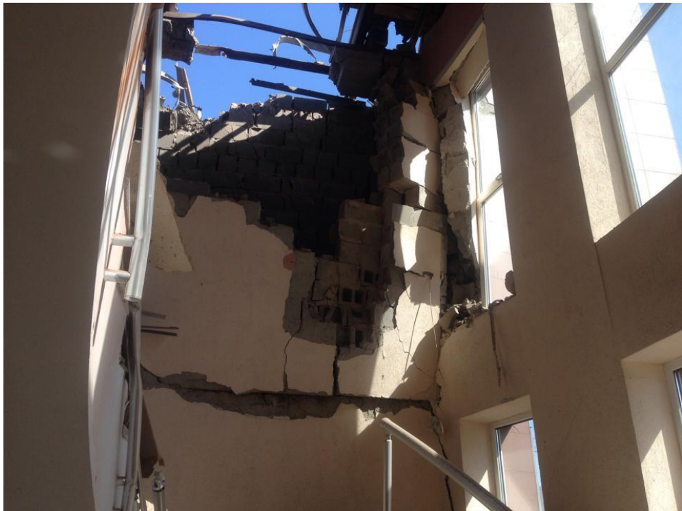
Fig. 19 – The roof of the prosecution office, destroyed by shell hit 9 47 .
