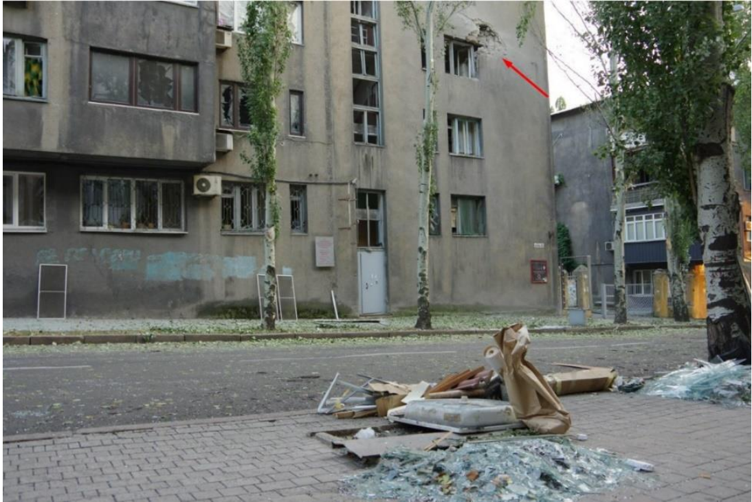
Fig. 2 – Shell hit (1) on the northern wall of a multi-storey residential building No. 58A in Artyom Str. Between the third and fourth floors 31 .
