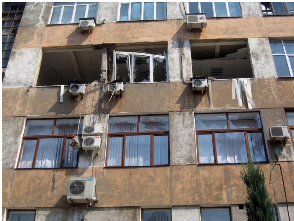
Fig. 11 – Shell hit (5) in the window at the third floor on the western side of the DonNTU educational building No. 1 40 .
