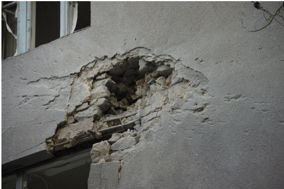
Fig. 3 – A hole formed on the building wall as a result of shell hit 1 32 .
