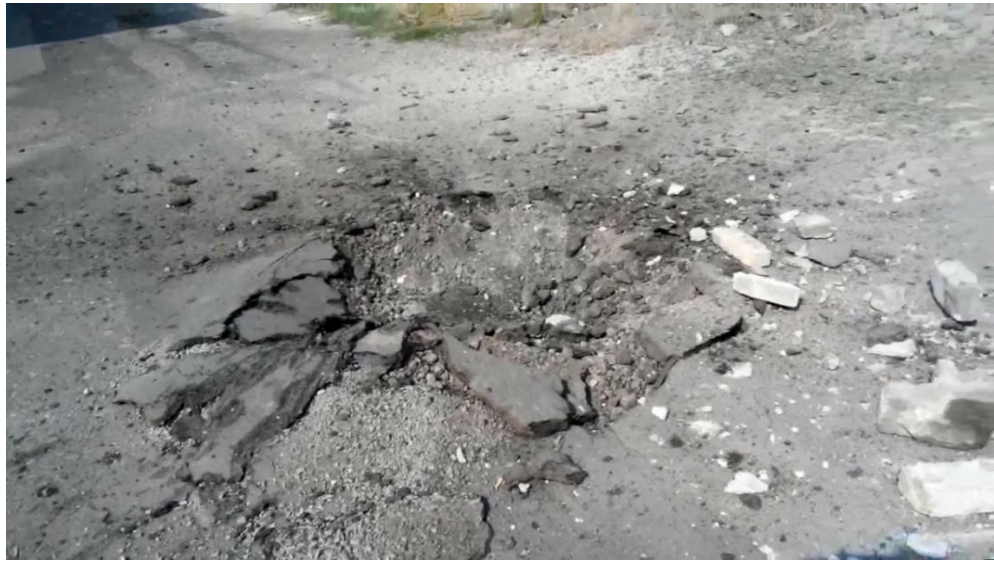
Fig. 10 – A crater created as a result of the projectile detonation about 60 meters west of the south-east corner of the DonNTU educational building No. 2 39 (shell hit 4).
