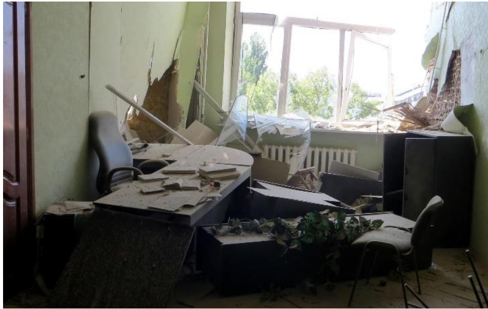
Fig. 12 – One of the DonNTU premises, destroyed as a result of shell hit 5 41 .
